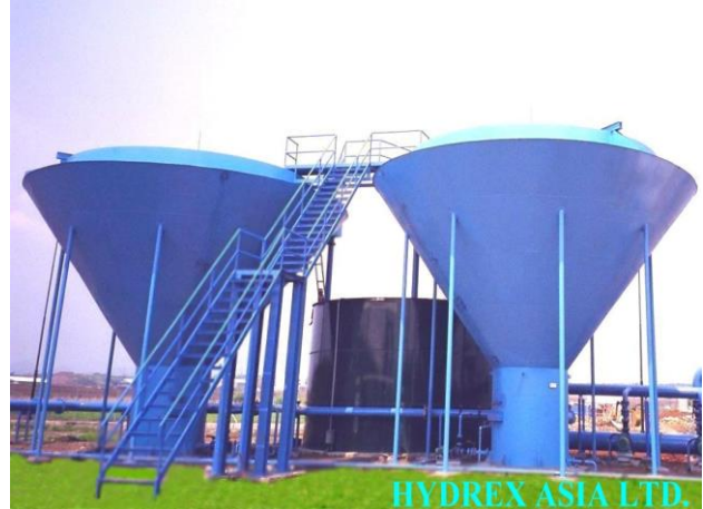
Two units 270 m 3 /hr total installed in Kawarang Industrial Park, for industrial and potable water treatment. (Java, Indonesia)
