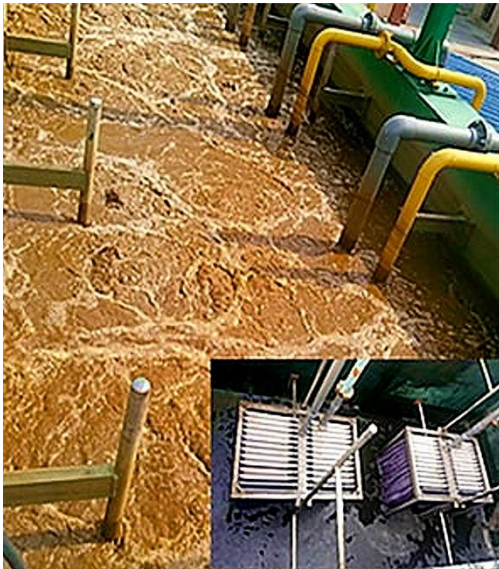
MBR in operation & drained down
