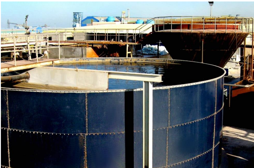
Anoxic Reactor and Hydrocone Clarifier
