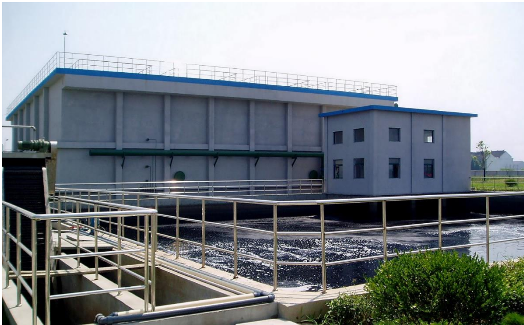
Equalization Tank and Anaerobic Reactor
