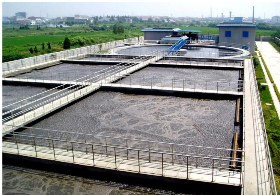
Aeration Tanks and Clarifier
