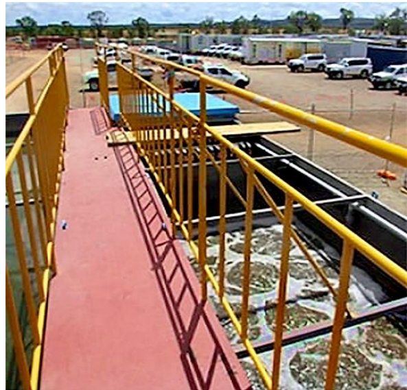
A Packaged MBR Plant
