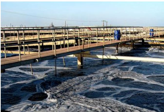
Oxic Tank with removal fine bubble diffusers
