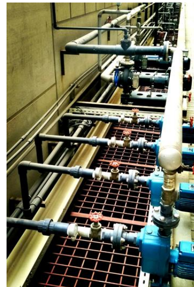
Some equipment mounted on top of tanks
