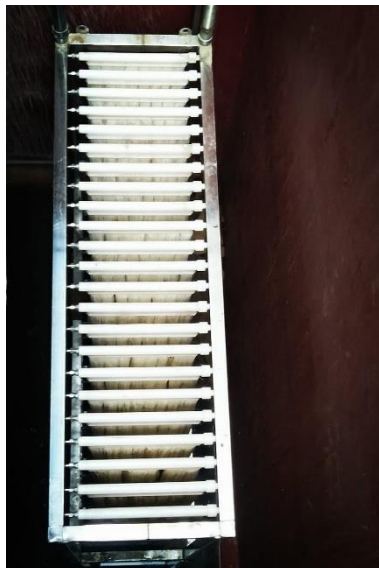
A membrane Cassette in the MBR tank
