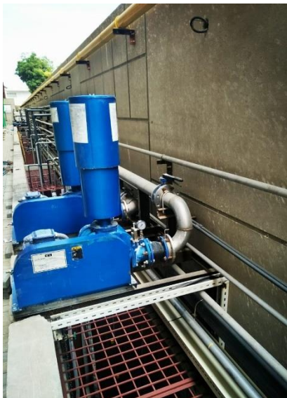
Air Blowers for MBR Air Scrubbing
