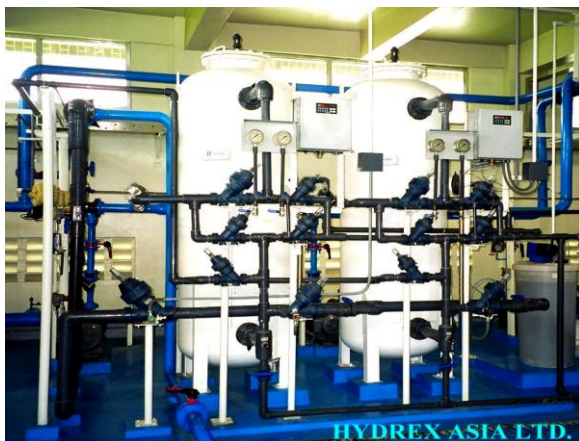
A fully automatic demin. train installed in a beverage factory for product manufacturing and for rinsing process.
