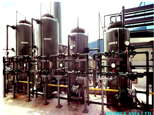
A two train demin. system installed in the Philippines steel coating plant for boiler feed water treatment.
