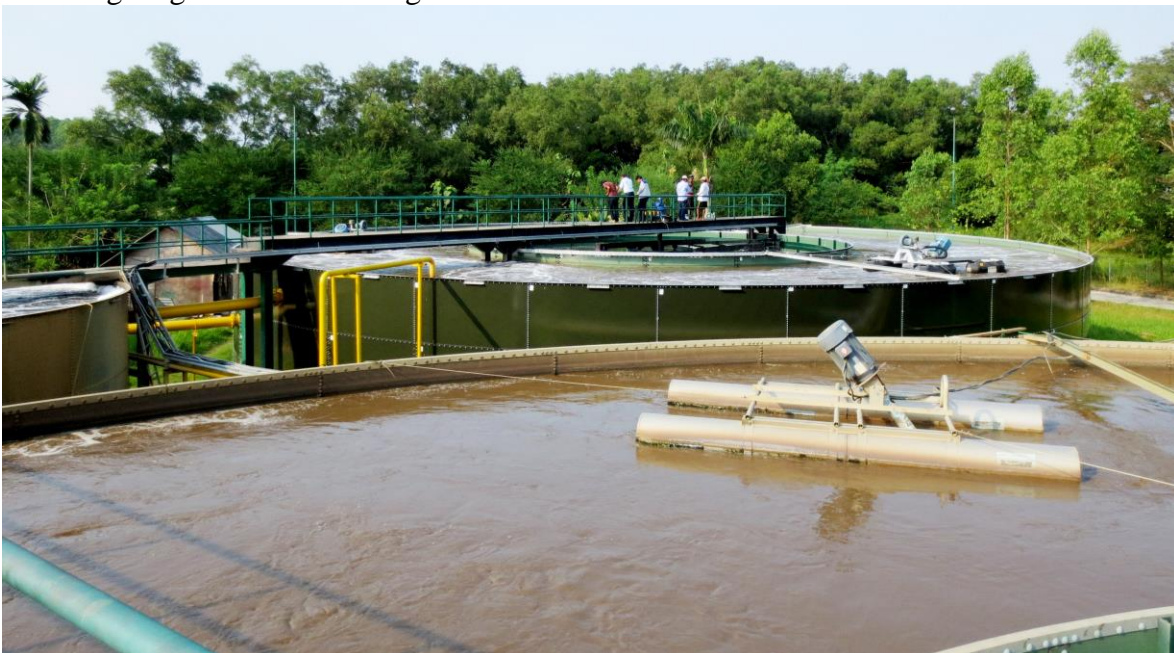
A- two (2) modules @20,000 population A/O Canal sewage treatment plant
