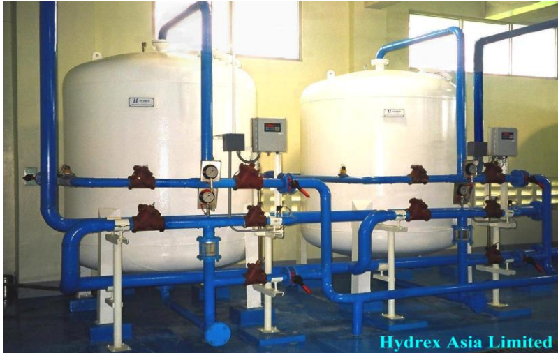
1.8m diameter automatic silica sand filters for a food processing factory.
