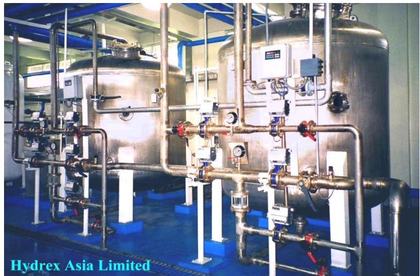
2.0m diameter automatic activated carbon purifiers with steam sterilization system.
