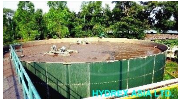
Aerobic Sludge Digester
