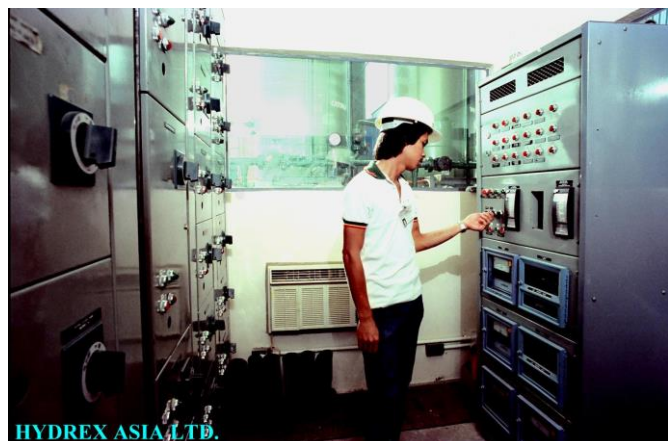
Central Control & Instrument Panels of a Wastewater Treatment System (above)
