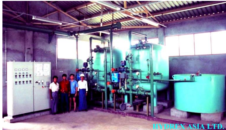
The fully automatic water softeners, 2m in diameter with resin regeneration equipment at the factory, plus the local crew.
