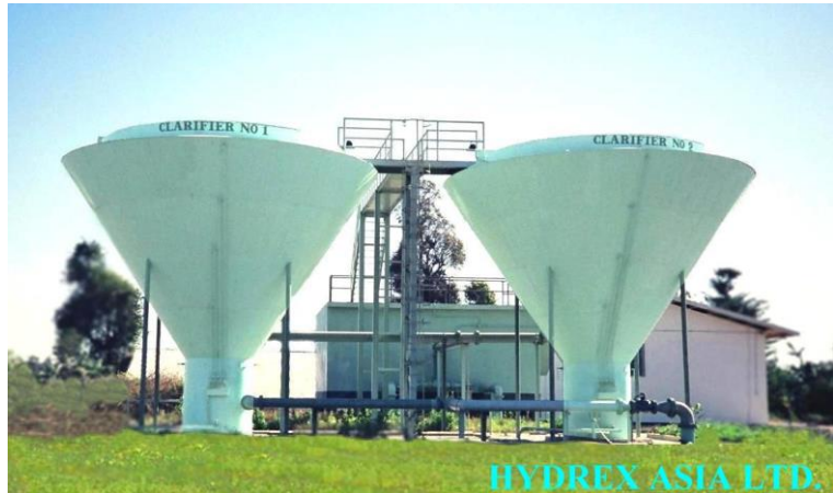
The 7m tall Hydrocone clarifiers that operate in parallel.
