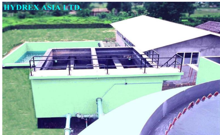
Looking down from the Hydrocones onto the riverside plant room, the gravity sand filters and the filtered water storage tanks.
