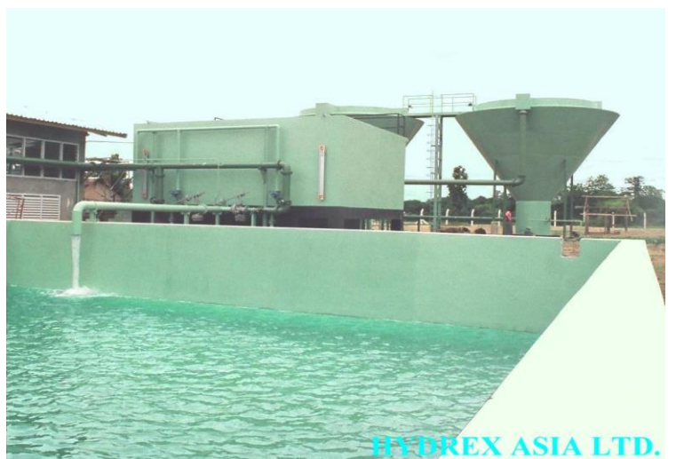
Clean, clear water in the filtered water tank
