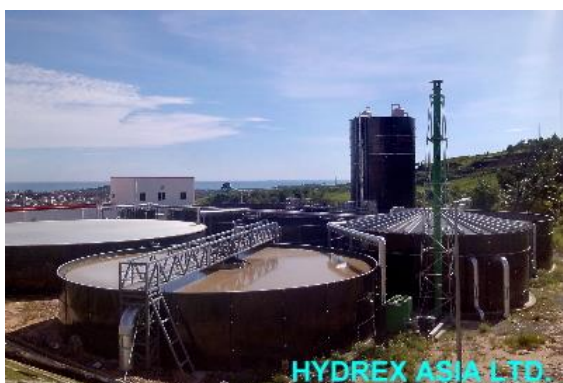
Glass Fused Steel Process Tanks
