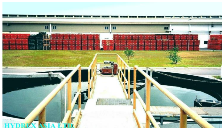
Wastewater Treatment System for Coca Cola's Bottling Plant in Hanoi, Vietnam
