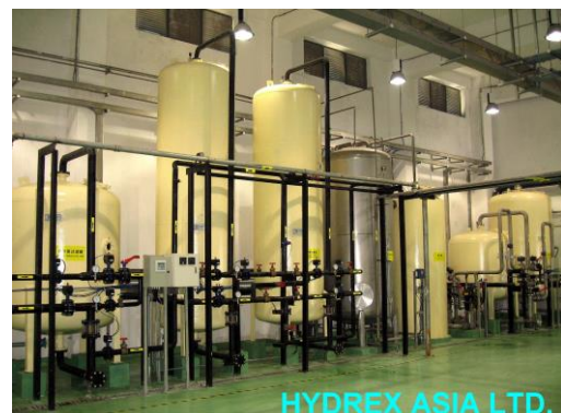
Tertiary Treatment and Color Removal System
