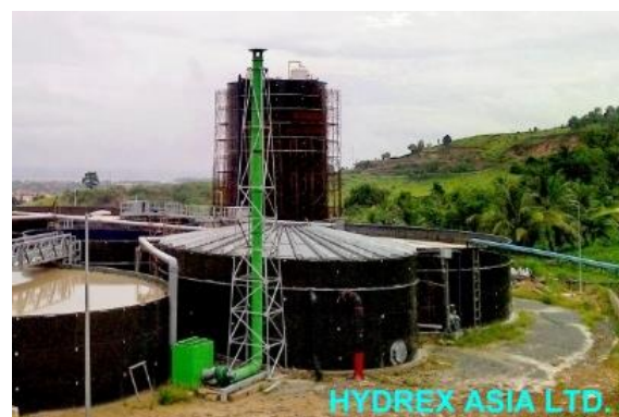
Glass Fused Steel Process Tanks with roof for the tall Anaerobic Reactor and Calamity Tank
