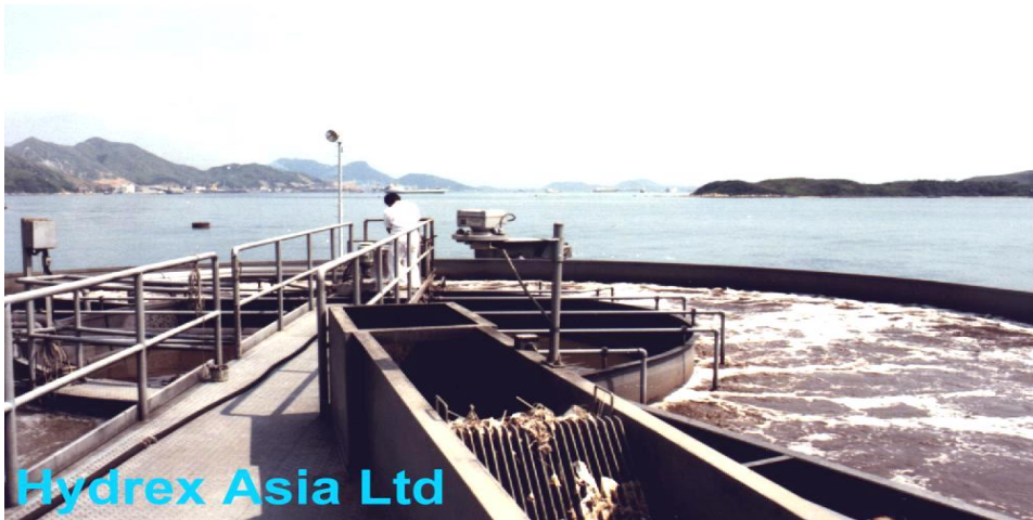
Cylindrical Wastewater Treatment Station for San Miguel Brewery, Hong Kong
